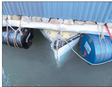
Afloat: A close-up showing the boat that has been lashed underneath the structure. Photo: BILL MOORE/FAIRFAX NZ
